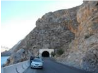
Rock fall section at the point of km 409 of the BO road, (installation of protection nets )
