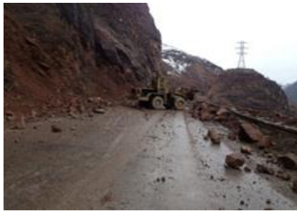
Rock fall section at the point of km 400 of the BO road (construction of a tunnel)
