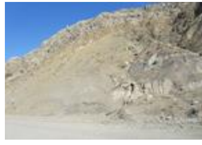
Landslide section at the point of km 451 of the BO road (installation of plumbers)
